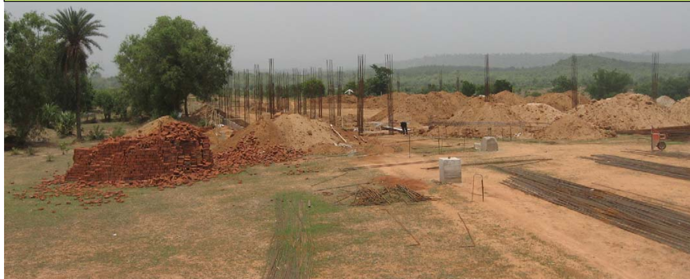
Construction works commenced toward the ECI Mission School building for the Malto children
